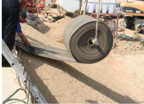
CC is rolled from the slope crest down the slope face, with 100mm overlaps between adjacent CC sheets.
