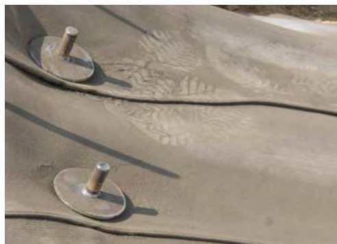
CC is fixed using short nails hammered into the soil. Other fixing methods such as drilled bolts can also be used if rock is present.
